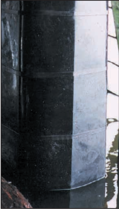
Hexagonal pile protected with SeaShield Series 100 system.
